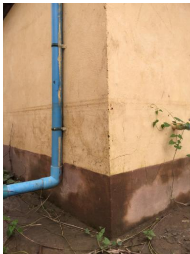
Water marks up to 1m above ground
