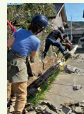
Dismantling and removing the concrete block wall of a home damaged in the Noto Peninsula Earthquake
